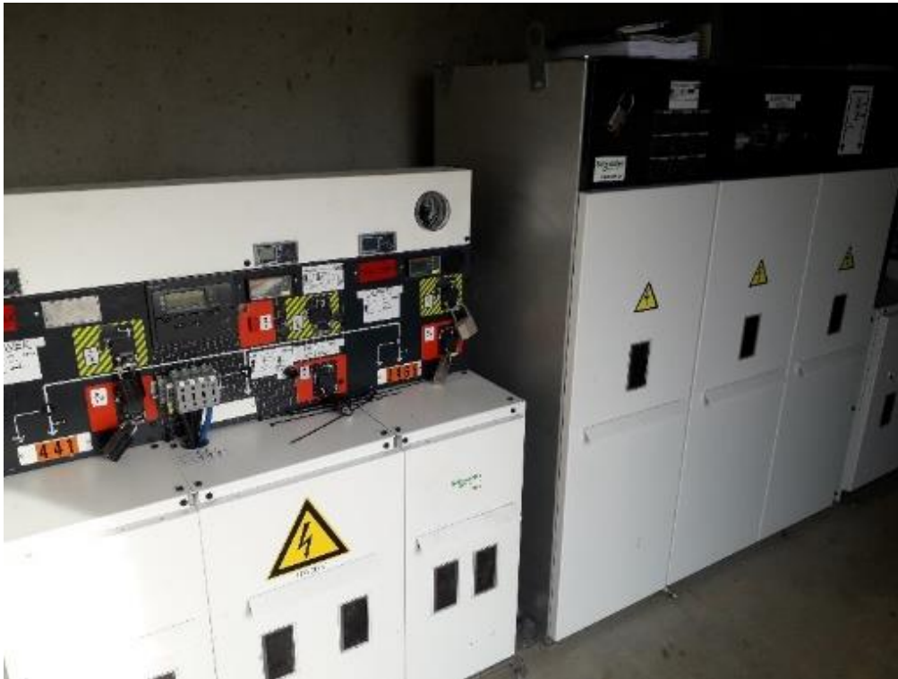
11 kV substation for a 800 kVA cogeneration unit.
